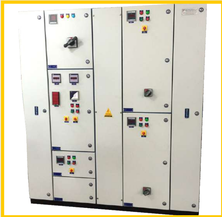
Fire Pump MCC
